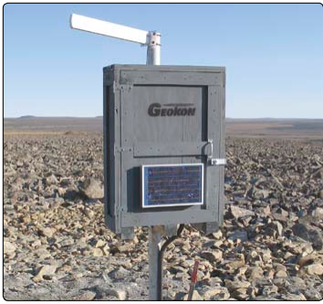
• Summer view of the Geokon Model 8025 Data Acquisition Station measuring a 70 m deep Thermistor String in mine tailings, located in northern Canada.*
