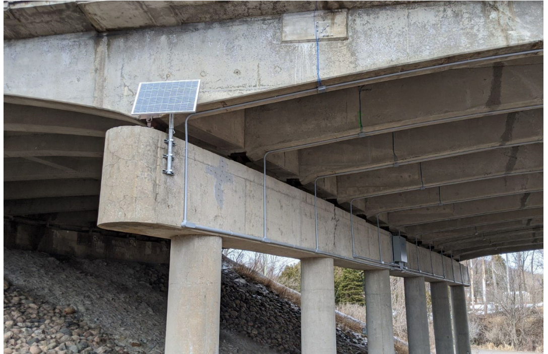
Structural Health Monitoring of an Overpass in Canada
