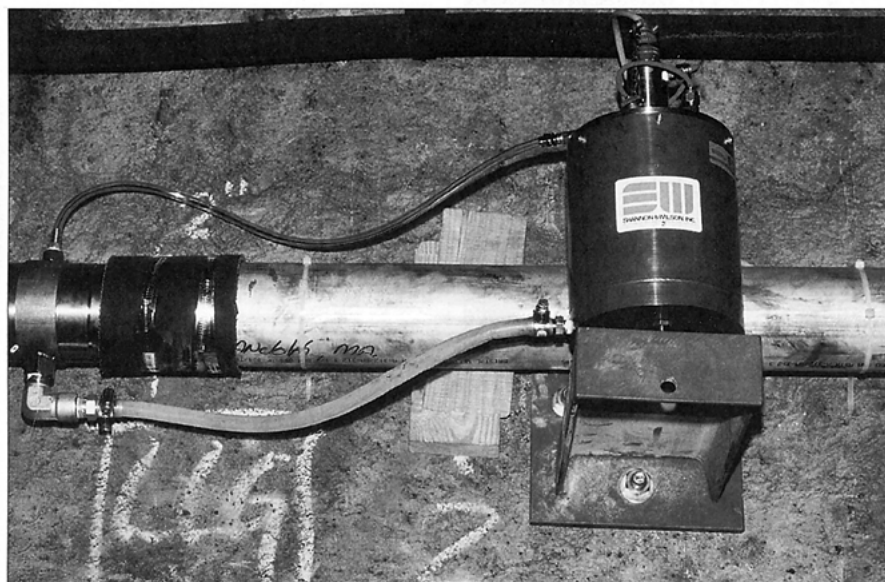
THE LIQUID LEVEL SYSTEM, MOUNTED ON THE WALL OF BOSTON'S RED LINE SUBWAY TUNNELS, MONITORS STRUCTURAL INTEGRITY WHILE A NEW TUNNEL IS BEING BUILT 1.5 M ABOVE.
