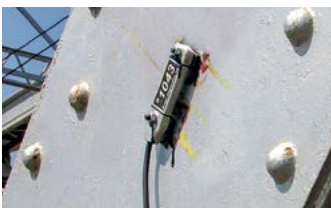
Model ST-350 attached to steel truss.
