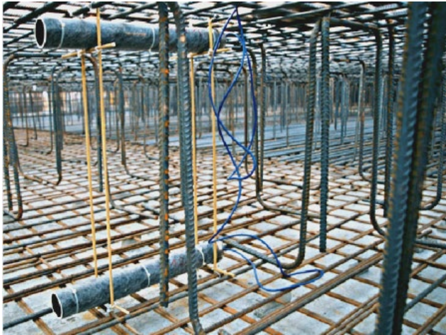
Figure 4 - Another typical stress meter installation
