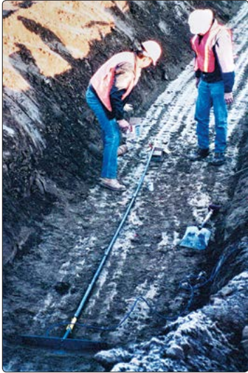
● Installation of Model 4435 sensors.
